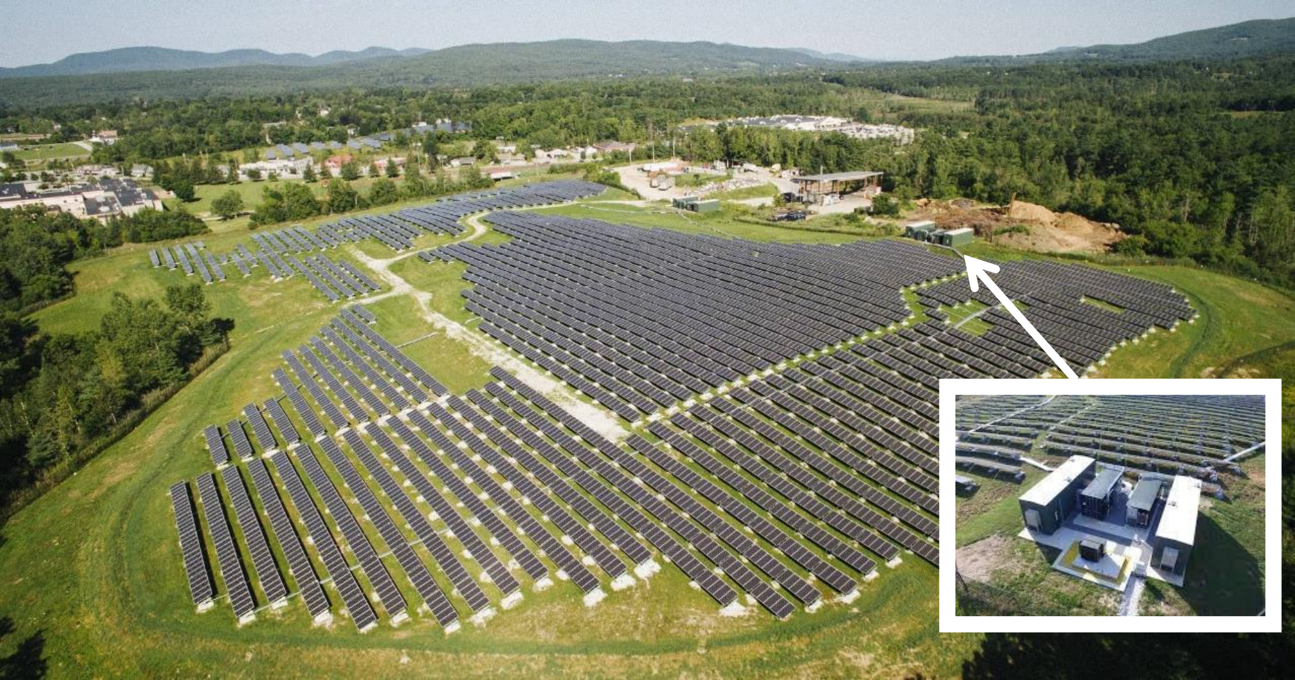
PV + Storage Microgrid supporting community resilience in Rutland, VT
