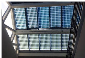
Internal view of PV systems @13P (about 30-kw)
