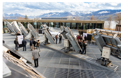
2020: The dual-axis trackers for solar collector testing, as installed in 1991. The people in the picture are participants of the annual Industry Day, during which SPF's 50 employees present their work.
