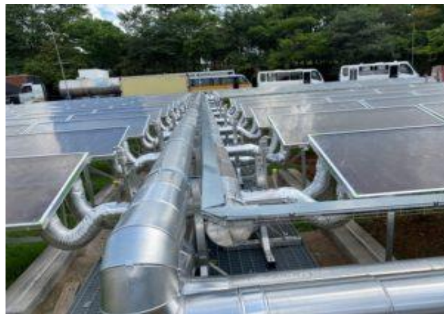
280 kW field evacuated flat plate collectors by TVP Solar in Brazil
