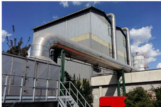
Waste heat recovery
